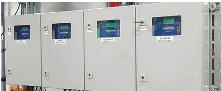
Commercial solar controller system at Fleurieu Aquatic Centre, SA
